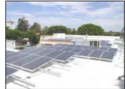
Solar panels on roof of 100 West Main Street.
