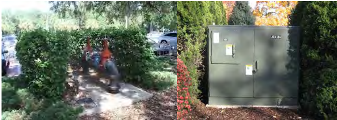
Utility equipment screened by landscaping
