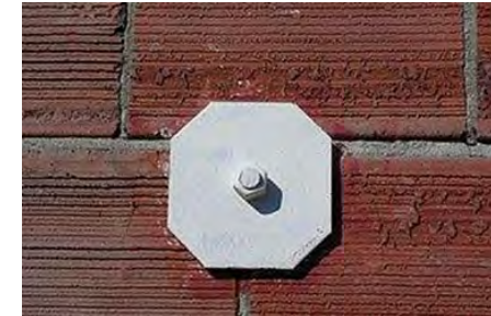
Poor example for seismic retrofitting a historic building.
