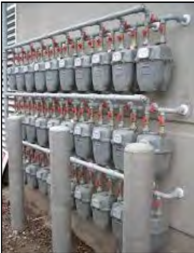
Bank of gas meters should not be visible from street and sidewalk.
